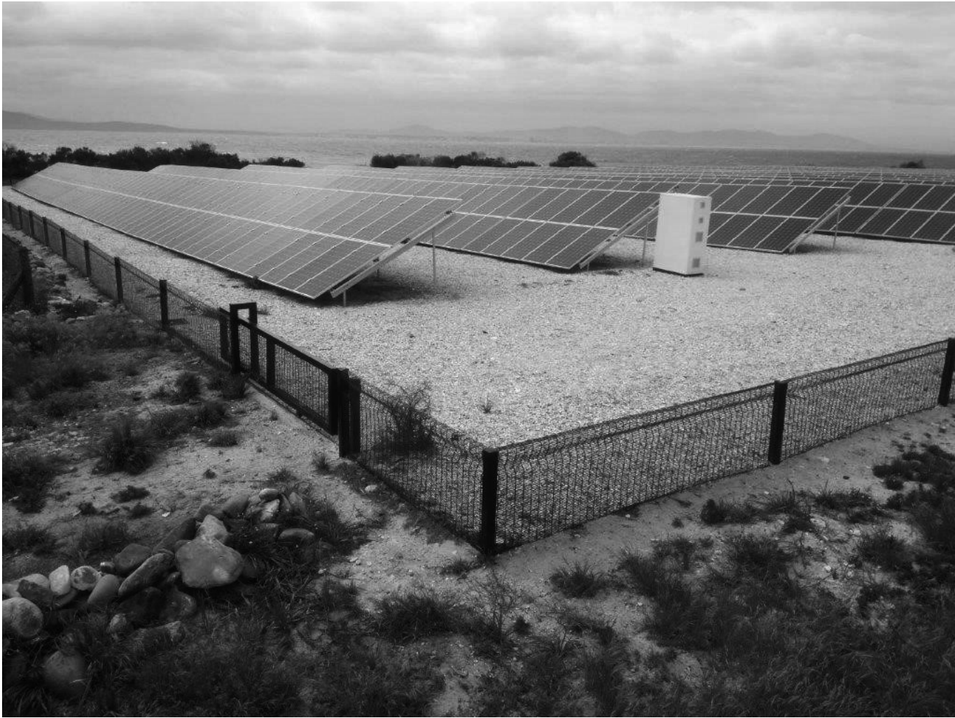
PHOTOVOLTAIC SOLAR PANELS. Robben Island World Heritage Site. Image: ©Pascall Taruvinga, 2018.
