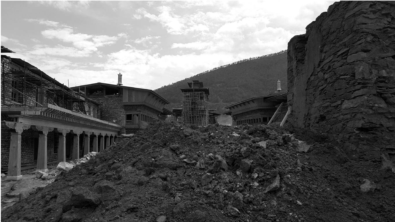
WANGDUAPHODRANG ZHONG, BHUTAN. Reconstruction following a devastating fire in 2012 through engagement of local craftsmen. Image: Rohit Jigyasu.
