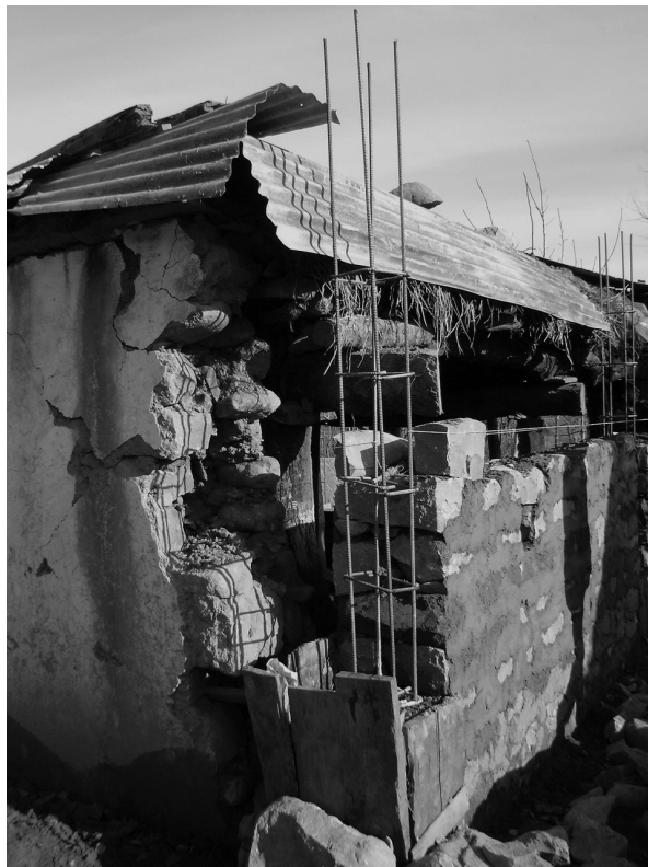
MARATHWADA, INDIA. Local masons carry out unsafe construction practices using new materials and technology because of lack of appropriate knowledge and unaffordability. Image: Rohit Jigyasu.
