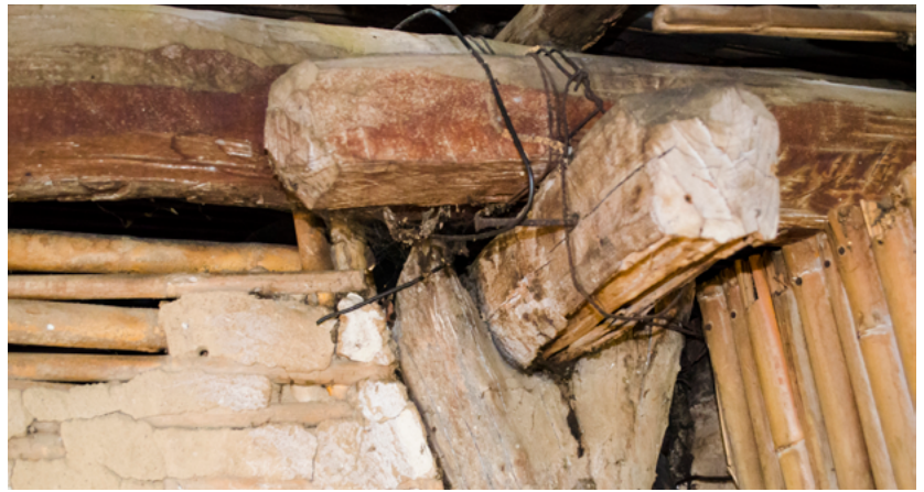
FIGURE 5. Detail of floor slabs underpinning the columns of the vertical structure and wire ties (Photograph: Antonio Flores, 2016).
