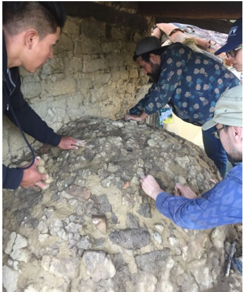
FIGURE 11. Restoration of a heritage oven during a workshop for conservators at the Escuela Taller de Boyacá, in Villa de Leyva, Colombia (Photograph: Luis Fernando Guerrero Baca, 2018)
